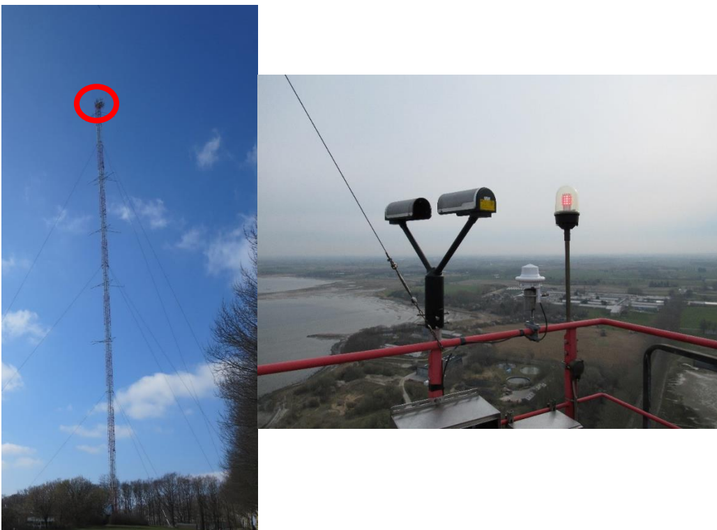
Figure 5: Disdrometer installation at DTU Risø campus (left) at the top of the meteorological mast (RTT) and (right) view from the top.
